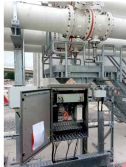
ICM monitor - GISmonitor outdoor installation
