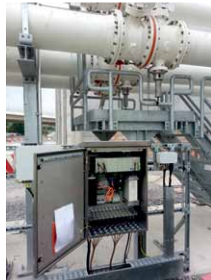
ICM monitor - GISmonitor outdoor installation
